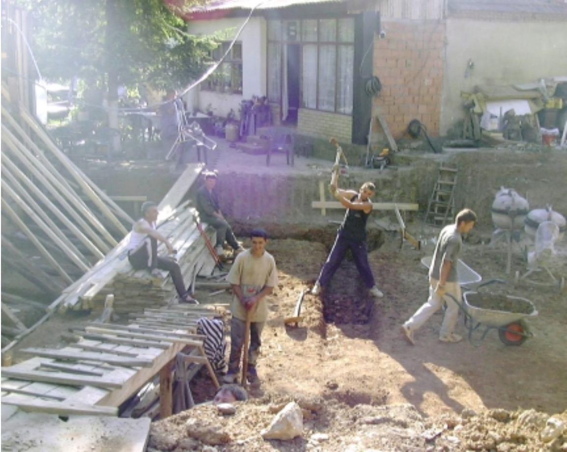
Rebuilding Kosovo - The author has never seen an area with more active construction going on! (Picture by Dr. Wendy Brown.)
